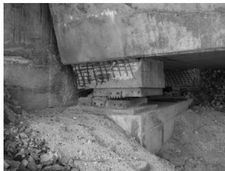
Damage to the abutment: offset of the hinge of the bearing part and damage to the abutment stone
