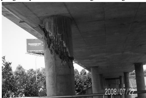
Mianyang Airport Terminal Bridge, bearing shear failure
